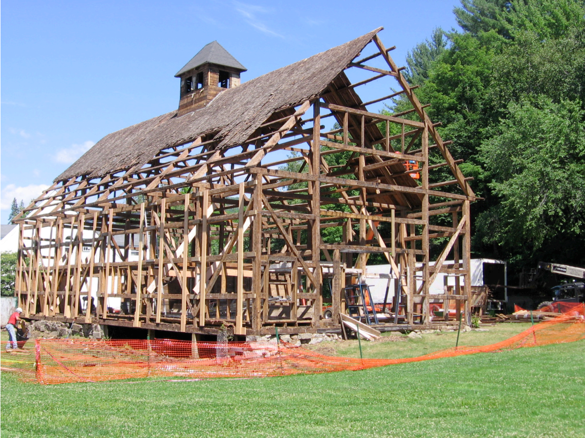
July 2008. Dismantlement begins. All the posts, beams, roof trusses, etc. are numbered for ease in reconstruction. The roofing, siding, windows, doors, all having been exposed to the elements, were discarded. The saved materials were stored in trailers.
